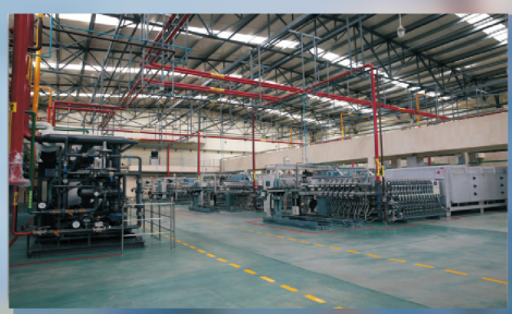
制粉车间 Powder process workshop
